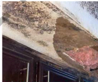
Mold - Lake growth was observed on the ceiling and wall sheetrock.
