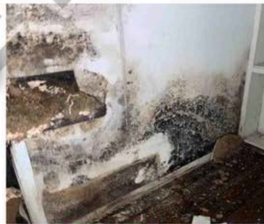
Mold-like growth was observed on the ceiling and wall drywall in this area.
