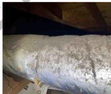
Mold-like growth was observed on the ductwork, and on the air handler cabinet.
