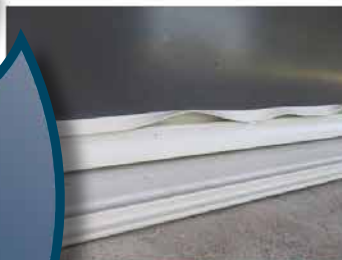
Buckled weather stripping at patio door.
