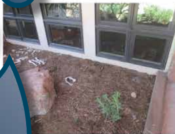
landscaping materials are in contact with the stucco wall coverings.
