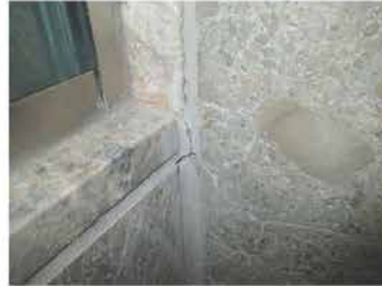
Cracked grout conditions outside of shower.
