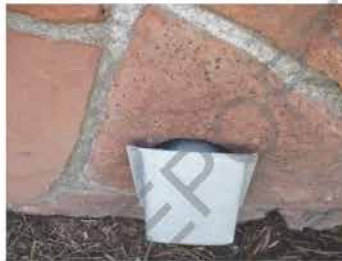
Unsealed penetration at vent.
