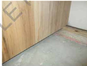
Water staining at the cabinet materials.
