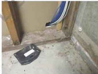
Water staining at the framing / wall.
