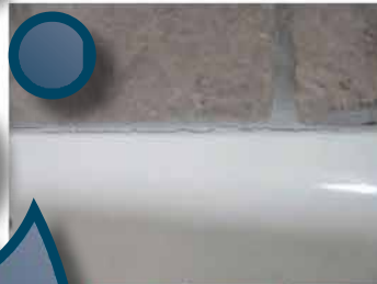
Cracked grout conditions in Shower.
