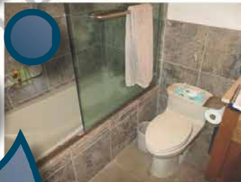
Mold-like growth on grout conditions in Shower.
