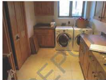
Water staining behind the washing machine and under the sink cabinet.
