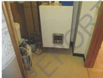
Water staining and mold-like growth were observed.
