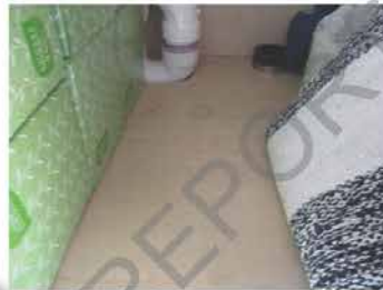
Surface staining at the cabinet base below sink.
