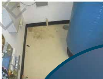
Standing water from the water
