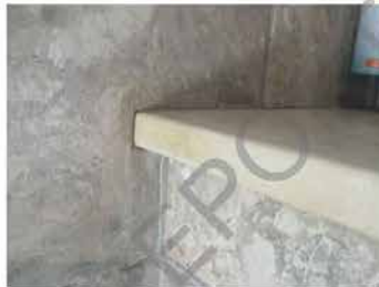
Unsealed penetration at shower seat / wall transition.
