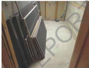
Water staining at the framing / wall common to the Basement SE Room.
