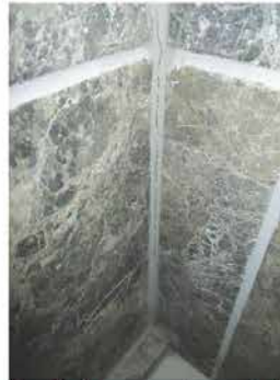
Cracked grout conditions in Shower.
