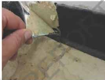
The water is tracking to the back wall, mold-like growth observed below the cover base.
