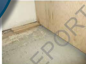
Water staining at the cabinet materials.
