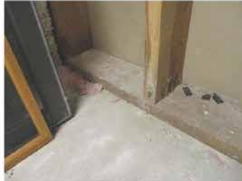
Water staining at the framing / wall.
