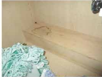
Water staining at the cabinet base below the sink.
