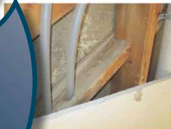
Water staining at the framing materials.
