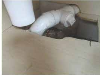
Water staining at the cabinet base below sink.
