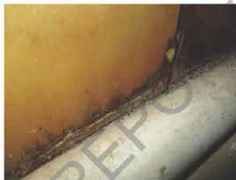
Mold-like growth at the Wall Paneling.
