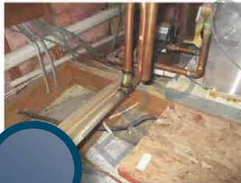
Water staining at the framing and vapor barrier.
