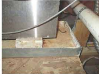
Corrosion and rust at equipment drain pan. It appears as if this overflowed at times and caused the water damage.
