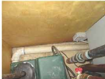
Water staining at the floor and wall materials.
