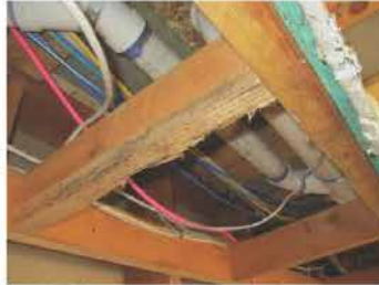
Mold-like growth at the Ceiling Framing.
