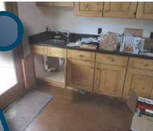
staining at the cabinet base below
