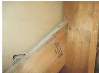
Mold-like growth at the Wall Framing.
