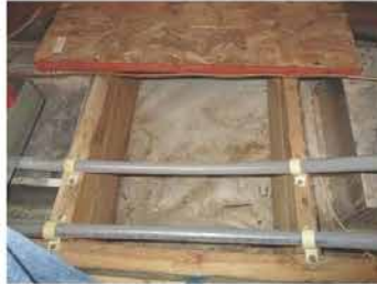
Water staining at the vapor barrier, this is believed to be the Master Shower ceiling.
