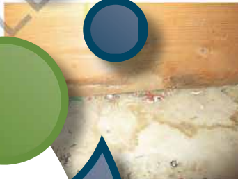
Water staining at the framing.
