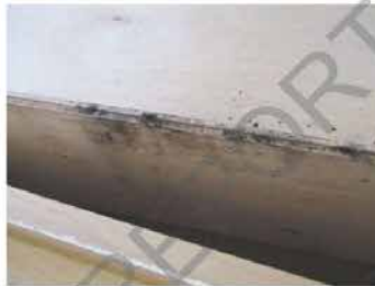
Mold-like growth at the Upper Cabinets, previously removed from the ceiling area.
