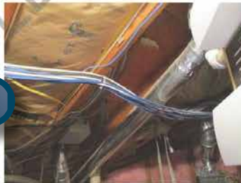
Missing insulation at roof.
