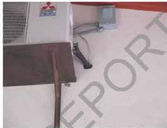
Unsealed penetration at HVAC lines.
