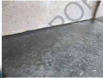
Cracked grout conditions behind sink.
