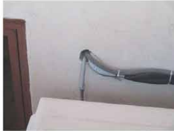
Unsealed penetration at HVAC lines.
