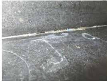
Cracked grout conditions behind sink.
