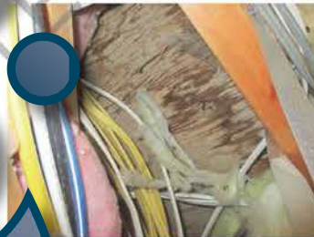
Staining at roof sheathing. Also, insulation in this bay.
