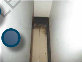
Water staining at the floor materials.
