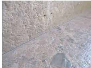
Cracked grout conditions at Tub area.
