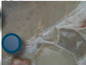
Cracked grout conditions in Shower.
