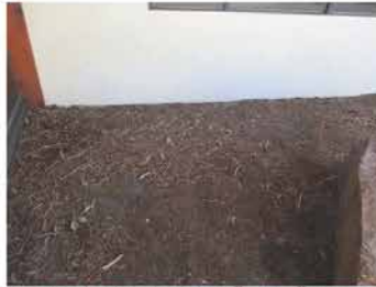
The landscaping materials are in contact with the stucco wall coverings.
