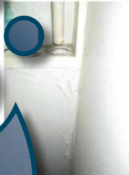
Water staining at the wall behind the washing machine.
