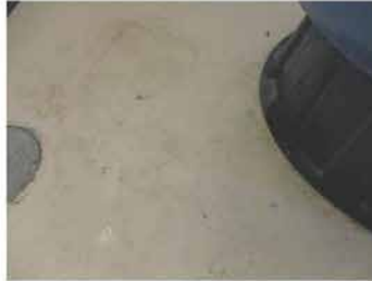
Standing water at the floor originating from the water vessel.
