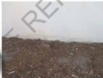
staining at the stucco wall
