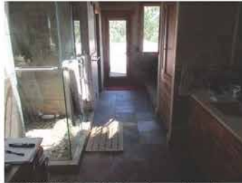
Mold-like growth was observed in the Master Shower.
