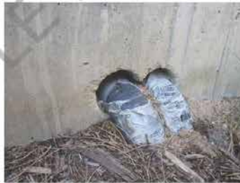
Unsealed penetration at equipment lines.
