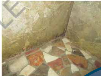
Mold-like growth at the Shower
