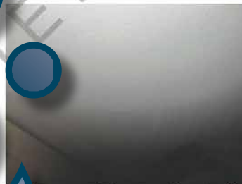
Water staining at surface of wall behind washing machine.
