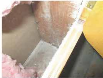
Water staining at the Baseplate common to the Closet / Basement SE Room.
