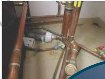
Water staining on the floor.
