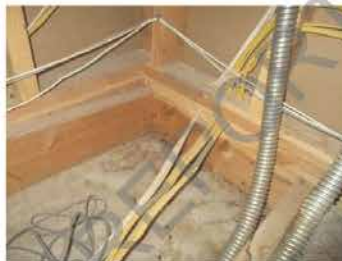
Water staining at the framing and vapor barrier.
