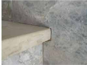
Unsealed penetration at shower seat / wall transition.
