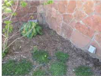
The landscaping materials are in contact with the stone wall coverings.
